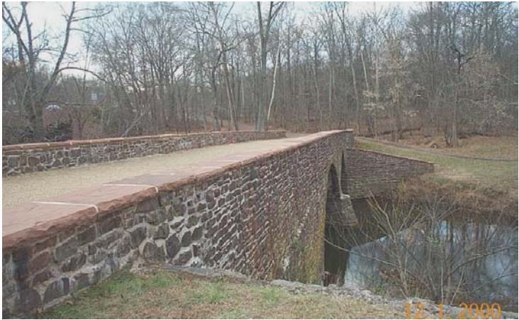
The Stone Bridge at Manassas National Battlefield Park in Virginia was restored to its original Civil War condition. The project was completed in 2000 with 80 percent Fee Demo revenue.
