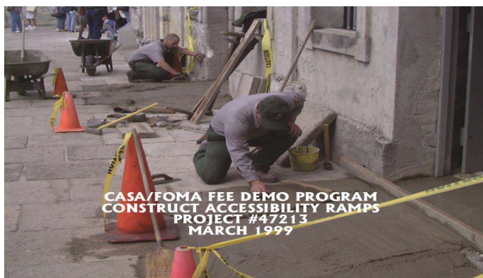
NPS facilities management division constructs and repairs handicap accessibility ramps at Castillo De San Marcos National Monument.
